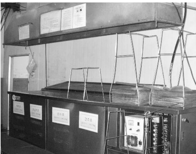
Figure 5. A case on the manual degreasing work by open top degreaser with a canopy type of ventilator
