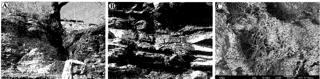
Figure 12. Biological weathering and a scanning electron microphotograph of bedrock under the Chokseongnu pavilion. (A) Structural deformation of bedrock by tree roots pressure. (B) Bryophyte appeared moisture-retentive area. (C) Rock damaged by hypha of lichens and roots observed under the SEM.
