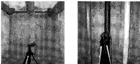
(b) Measuring photograph of horizontal branch pipe (c) Measuring photograph of riser pipe
