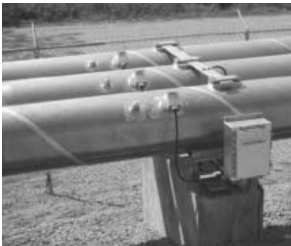
6-27 | Gas Density Monitor
