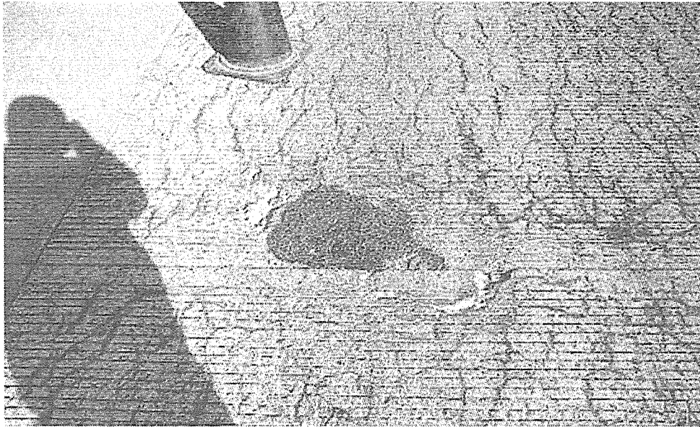
<사진 2> ASR Distress in Express Highway
