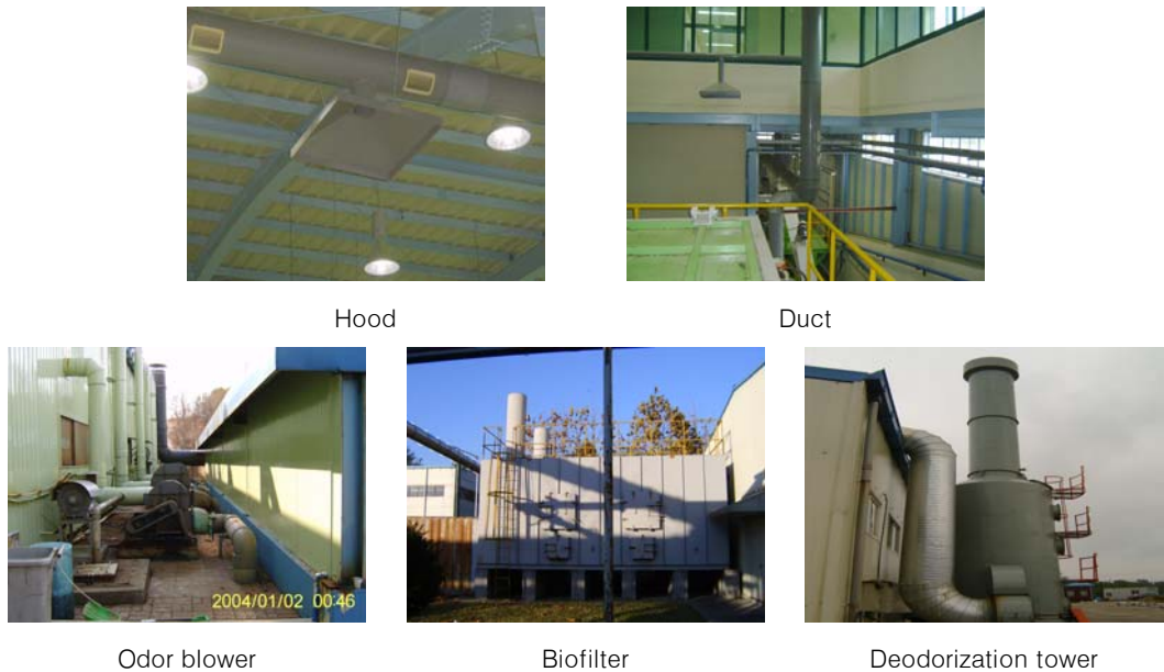
[Fig.8] Foodwaste treatment facilities in odor control installation.
