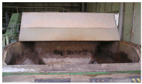
Closed Input installation
