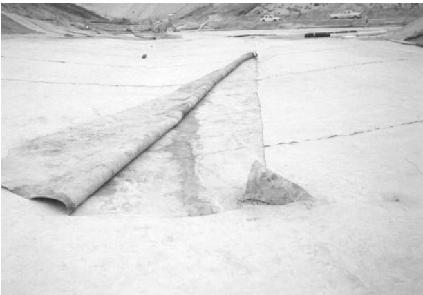
Fig. 2. Layer of hydrated bentonite on top of geomembrane on cell base after removal of overlying sacrificial geomembrane.
