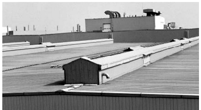
(b) Gravity ventilator installed on the top of industrial building
