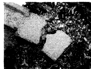
(c) Destroyed cap concrete
