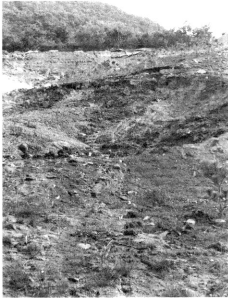
Figure 2. Tension crack of survey area.
