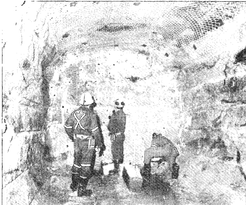
Fig. 9. Mining crews loading full-face blast round on the 420 Level of the URL.
