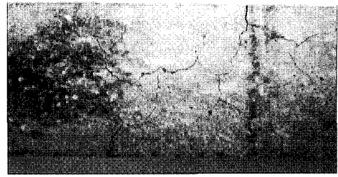
Fig. 12 Cracks caused by alkali-silica reaction of crushed stones used in the experiment
