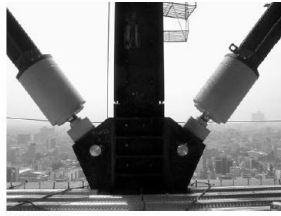
FIGURE 9 TAYLOR DAMPER INSTALLATION, LONG WALLS
