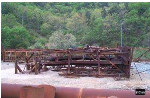
Fig. 10 View of set(up) and overturned(down) steel structure
