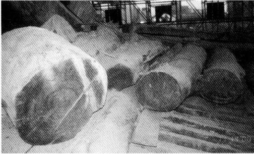
Fig. 3. Roof-packing logs of Keunjeongjeon Hall, where fir logs were frequently found.
