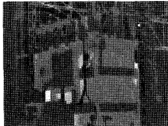
b) Electrical Systems
