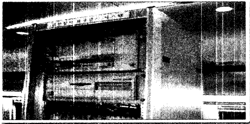
Fig. 5. Receiving part of telemetry and VXI processing system
