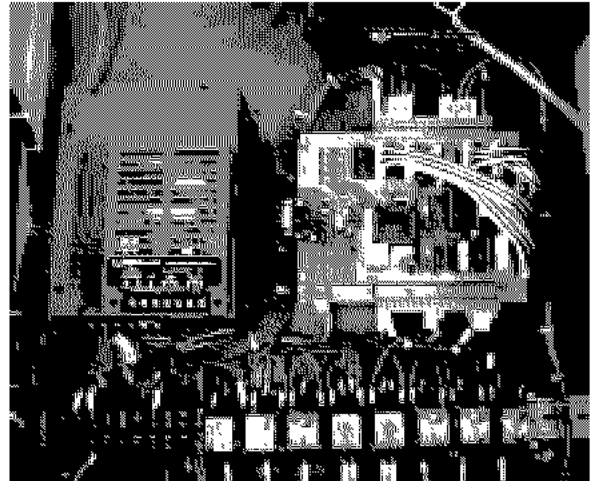
Fig. 8 80C196KC board in switchboard
