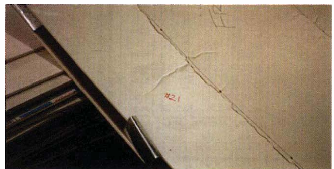
Fig. 6 Collapse of wallboard
