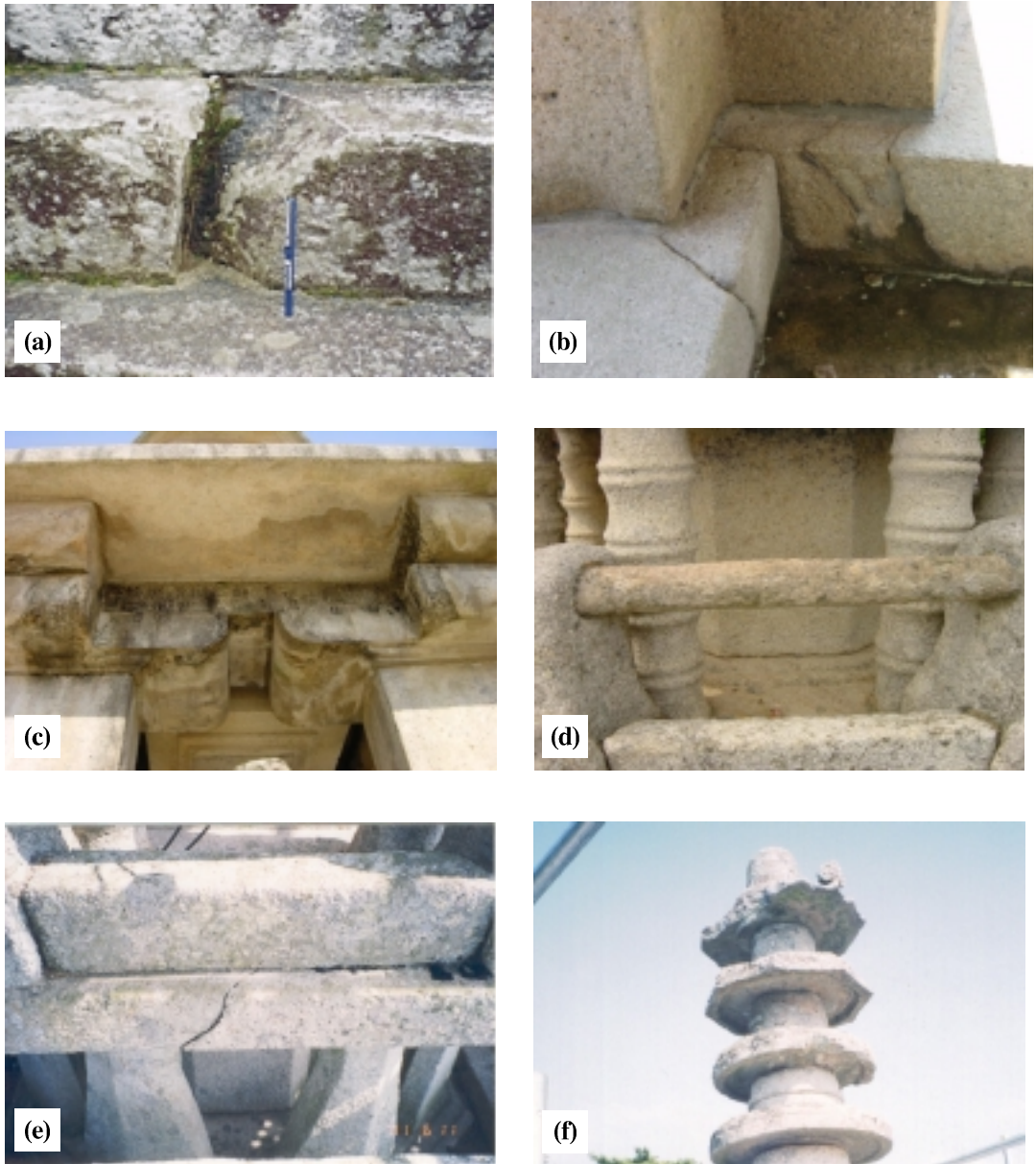
Fig. 2. Damage conditions of Dabo Pagoda; (a) a broken plane at a stairway, (b) fractures at supporting blocks on the platform due to unequal weight, (c) severely weathered cornerstones under the Kidan Gapseok, (d) a severely weathered parapit on the second floor, (e) a fracture of the first floor Gapseok, and (f) a broken plane at at Bogae.
