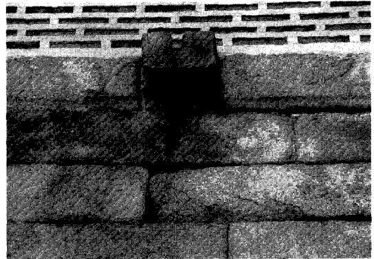
Fig. 14. Surface exfoliation and breakout by the differential load at the left-uppermost, east side of the north wall.
