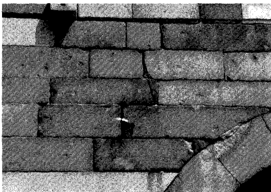
Fig. 13. Cracks and exfoliation by the differential load and edge-breakout at the right-uppermost, west side of the south wall.
