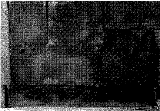
Fig. 15. Edge-breakout on the rocks at the east wall of the inner side of the gate.
