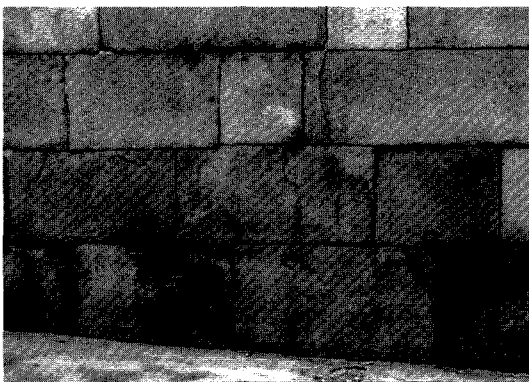
Fig. 10. Exfoliation and cracks by the onion structure at the lower-most of the central part, west side of the north wall.
