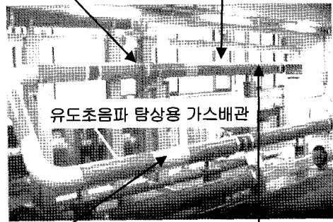
Wall thinning (taper) Flat bottom hole
