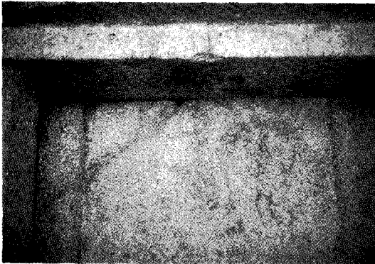
Fig. 12. Front of the seat; cracks and crack zones.
