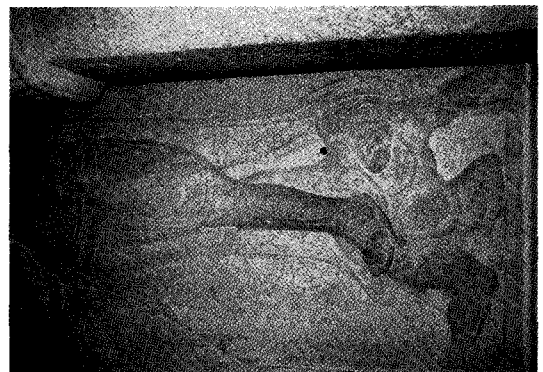
Fig. 10. Left 7 face of the fore-room: large cracks(left and right sides) and crack zone(width 0.5-3.0 cm at right lower part).
