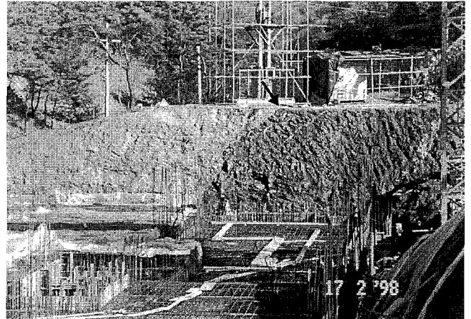
Photo. 1. The photograph of the neighborhood of station #11, profile Line 2. The arrow indicates the fault predicted by array CSAMT survey.
