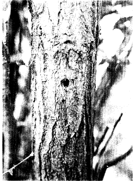
Fig. 1. Bark split from the injection wound on the stem of chestnut tree.
