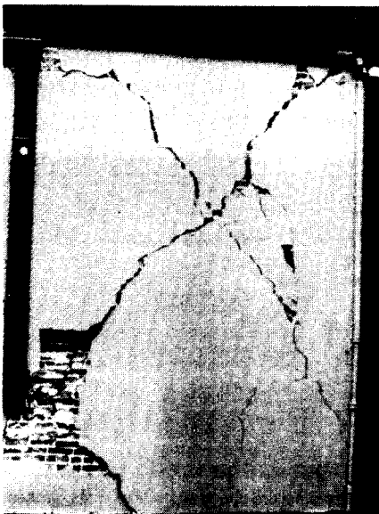
Photo.2 In-plane shear failure of URM masonry wall (Santa Cruz, Loma Prieta Earthquake)
