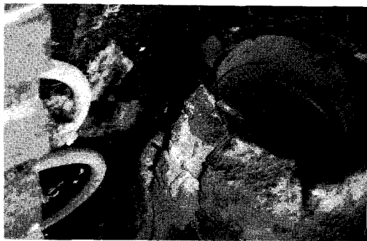
Fig. 1. Status of Hi-Alumina cementless castable in burner after 60 days.
