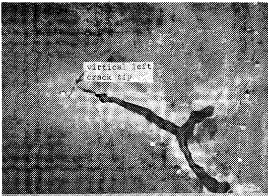
(b) Vertical left crack
