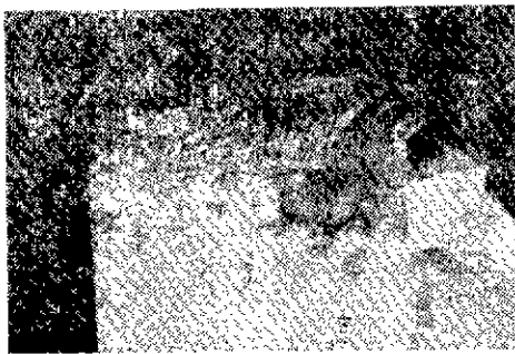
Fig. 2. Silica brick cracked by spalling after 98 casts in an arc-furnace roof. The major spall crack parallel to hot face has opened up sufficiently to permit metal and slag to enter.
