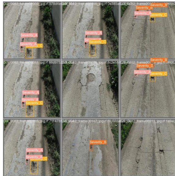
Figure 4. Result of pothole detecting based on guideline
