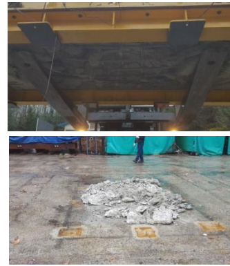
Fig. 4. Damage and deformation of concrete pad.
