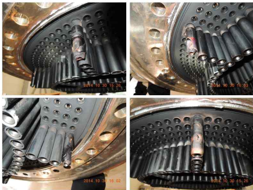
Fig. 5 Damage of Periphery Baffle Injectors
