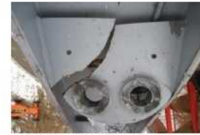
Fracture of steel member
