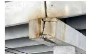
Fracture of concrete member
