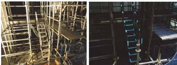
FIG. XIII Normal condition (left) and Switch off Power Supply near staircase of underground caisson works
