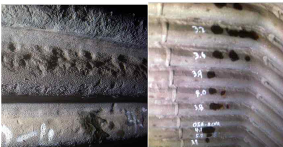
Fig. 4 Tube corrosion status & measurement point
