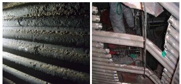
Fig. 2 Tube corrosion and maintenance
