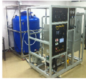
Submerged UF (Ultra Filtration) system
