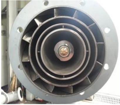
Fig. 3 Picture of burner exit
