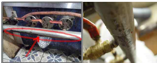
Fig. 2 Corrosion of manifold
