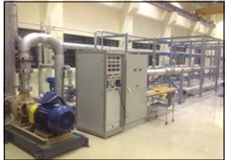
Fig.1 Picture of Test System: pump and controller
