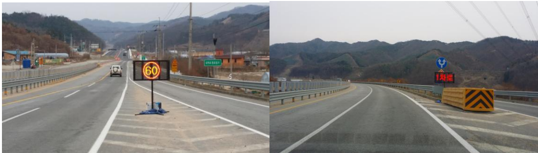
Figure 2. PVMS employed in the beginning and ending points of the work zone
