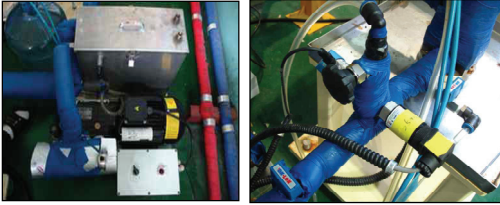
Figure 3 Pump and valves
