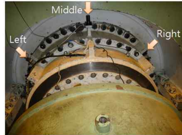
Fig. 4 The measurement locations on the generator endshield
