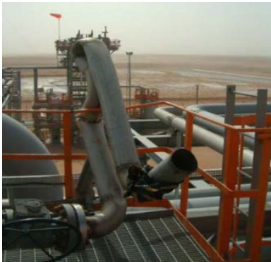
Figure 1 Gas flare header rupture
