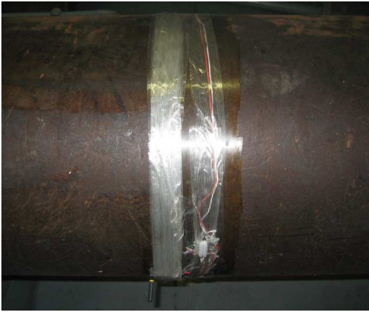
Fig.15 Telemetering System at Inter-Shaft
