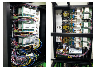
Fig 6 Photo of power stack
