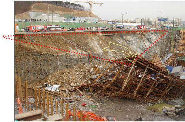
Figure 1. A case of earth retaining wall failure
