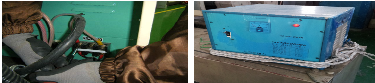
Figure 1. Contact failure of terminal block & installation failure
