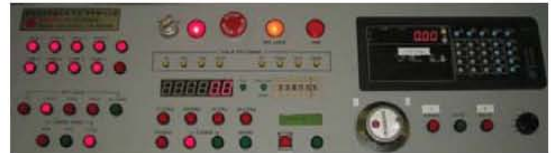
Fig. 2. Control Devices of Control Console.
