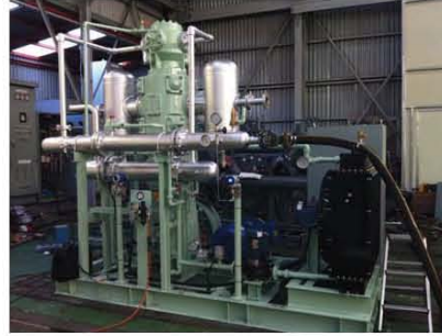
Fig 1. Argon Purifier Compressor.
