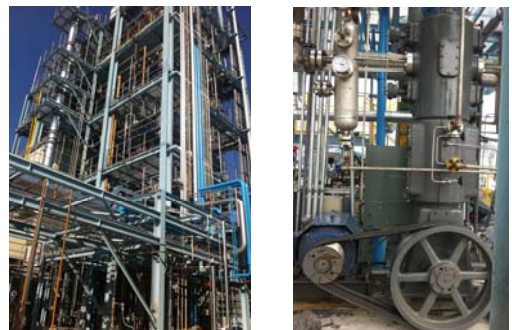
Fig. 1 Structure & Reciprocating Compressor
